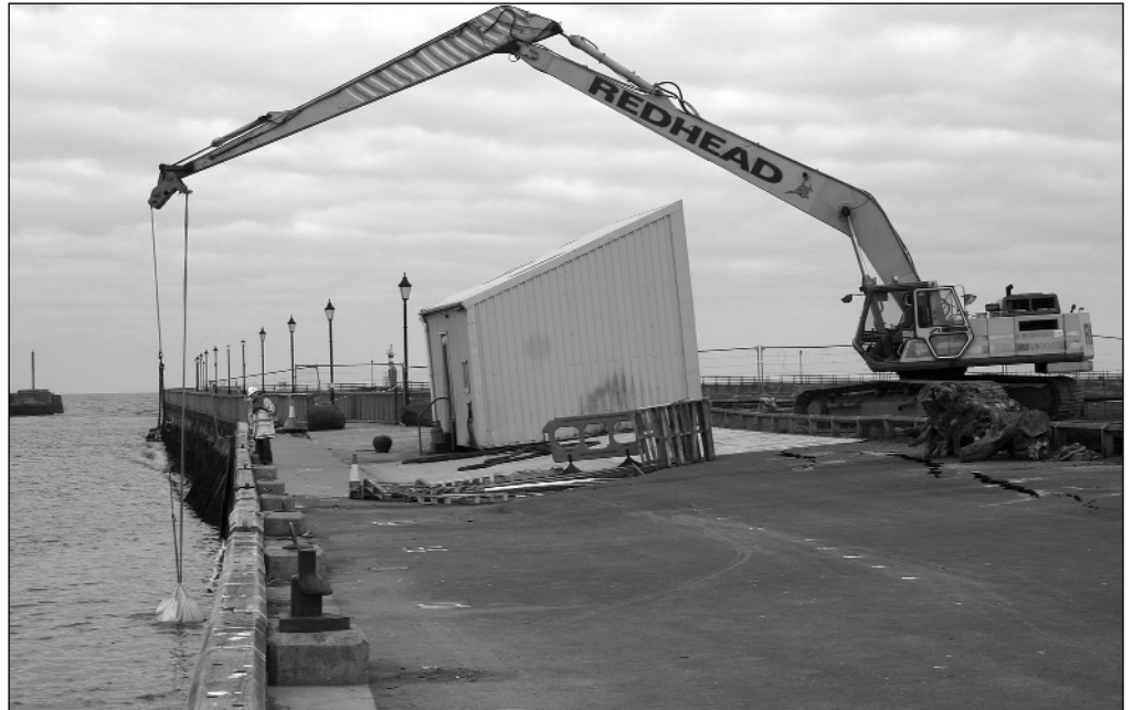
A crane positions bags of "rock armour" in front of the damaged area of the harbour. The cracks and subsidence required an emergency operation to empty out the oil store (centre).
